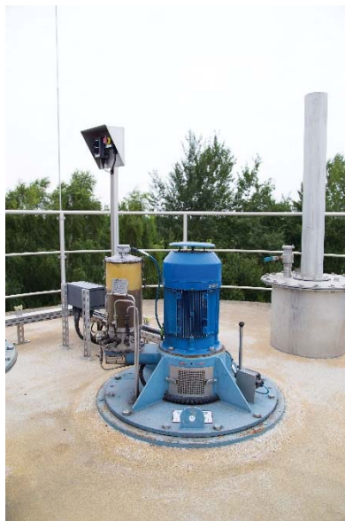
Stirrer digestion tower with central lubrication
