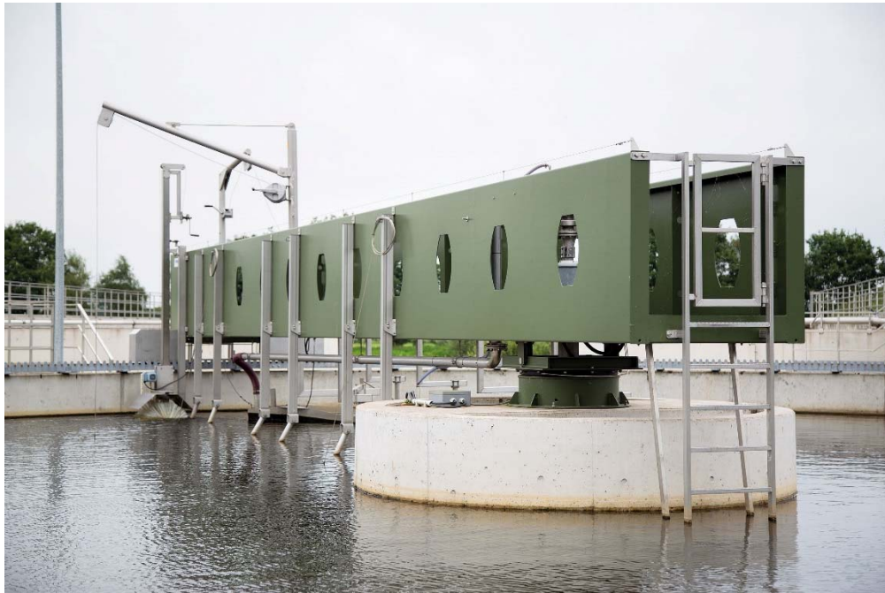
Secondary clarifier and round cleaner
